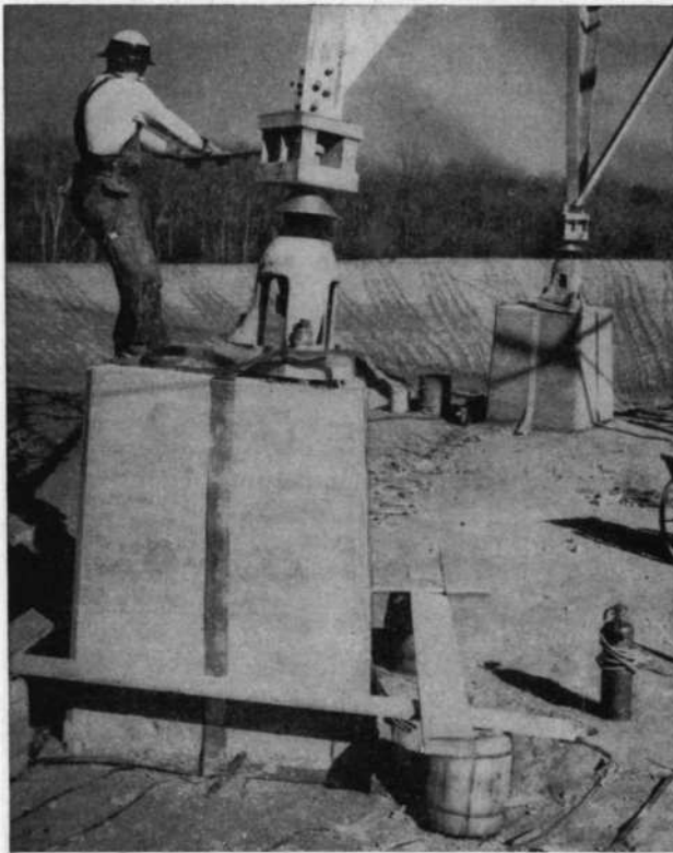
FIG. 2.56. Base of a self-supporting broadcast radiator during construction. Notice tractor and plow tracks in background where ground wires have been plowed into the soil. (Photograph courtesy of National Broadcasting Company.)
